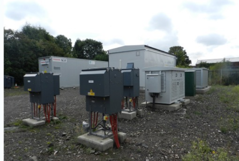
2MW grid connected test facilities
